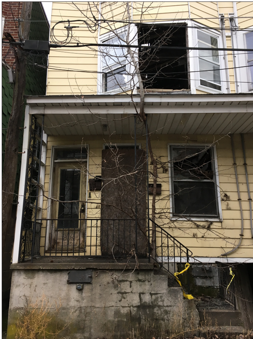
12. A tree grows upwards from a concrete porch.
